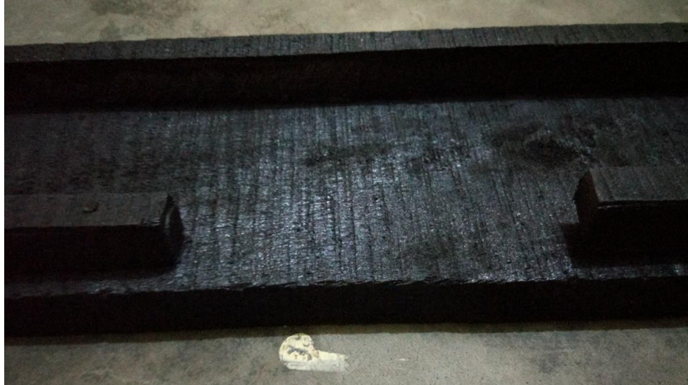
Fig 4.6: Faulty section of the track
