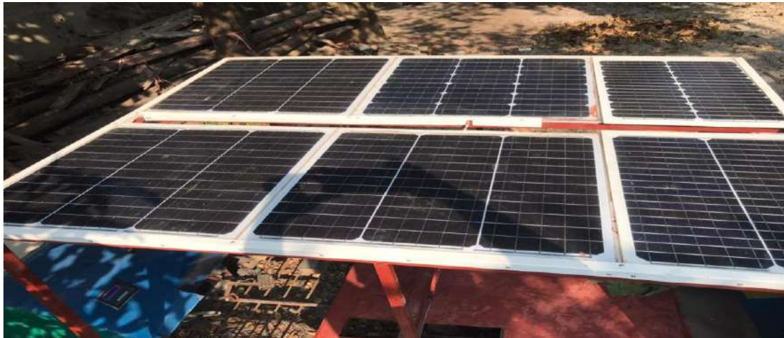
Fig. 5.2: Solar Panel Setup
