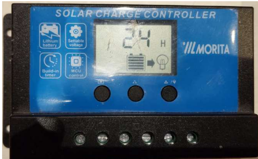
Fig. 4.14 Power Consumption From Solar Panel
