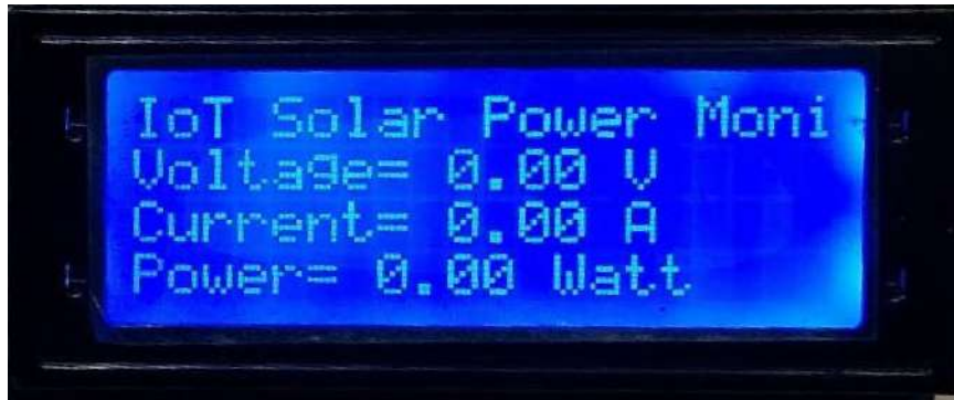
Fig. 4.18 When Load not Connected, value of Voltage, Current and Power
