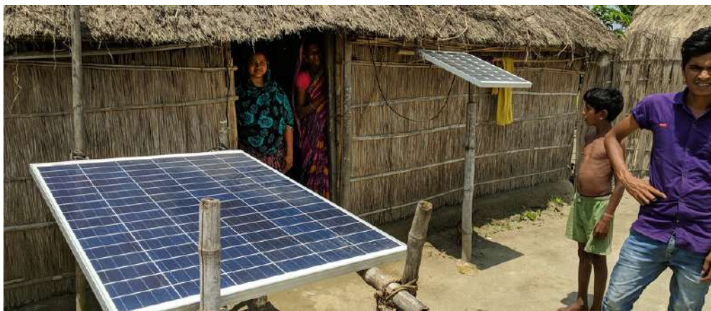
Fig. 2.6 A SHS in a rural area of India [5]
